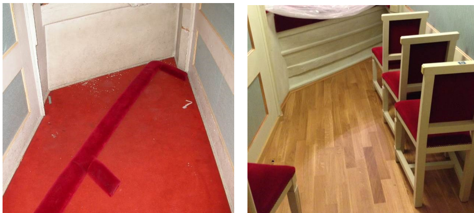
Figure 1: Teatro Zandonai, Rovereto: the interior of a box prior to renovations (left) and after refurbishment (right). Note that a panel was removed from the box fence to revamp the original lathed structure. Moreover removing the carpeted floors is often intended as a philological approach to the heritage, since carpets were introduced in earlier renovations, when sometimes theatres were used also as cinemas especially in smaller towns [5].
